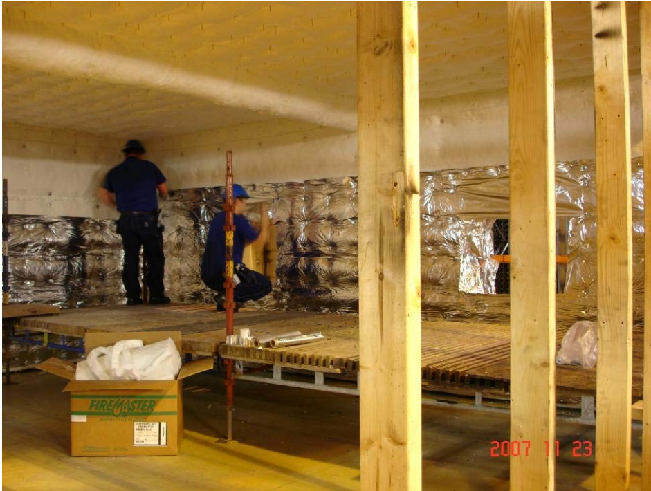
Figure 4-12 Interior FRD 60 insulation of the composite, before cabin construction. Note the stiffener at the ceiling (“upper deck”).
